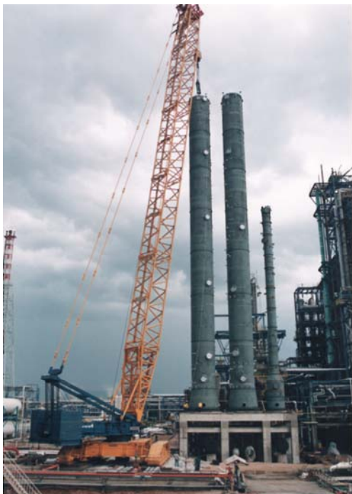
2 P/P Splitter Towers (HELPE)
