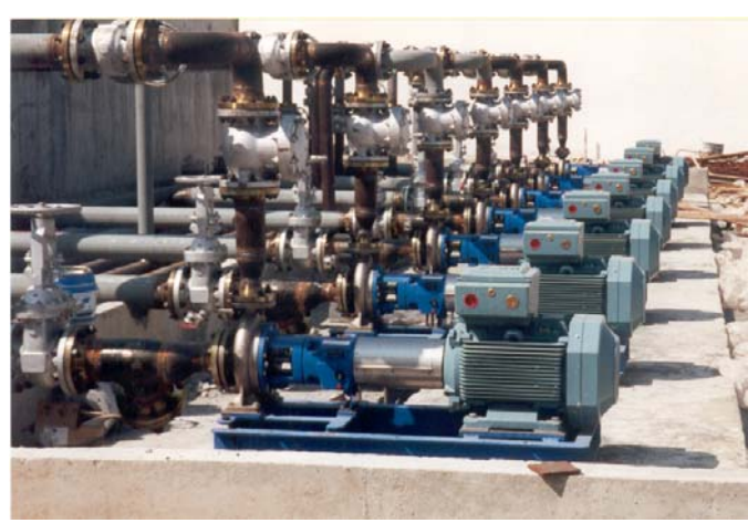
Fuel Pump Station for a Tank Farm (GLOBAL ALBANIA)
